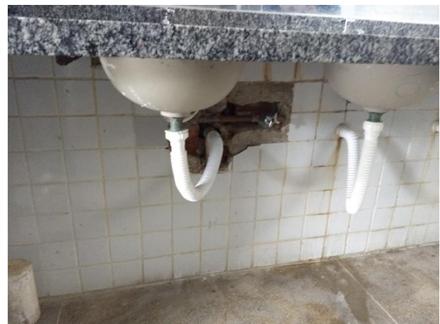
(b) Reforma incompleta
